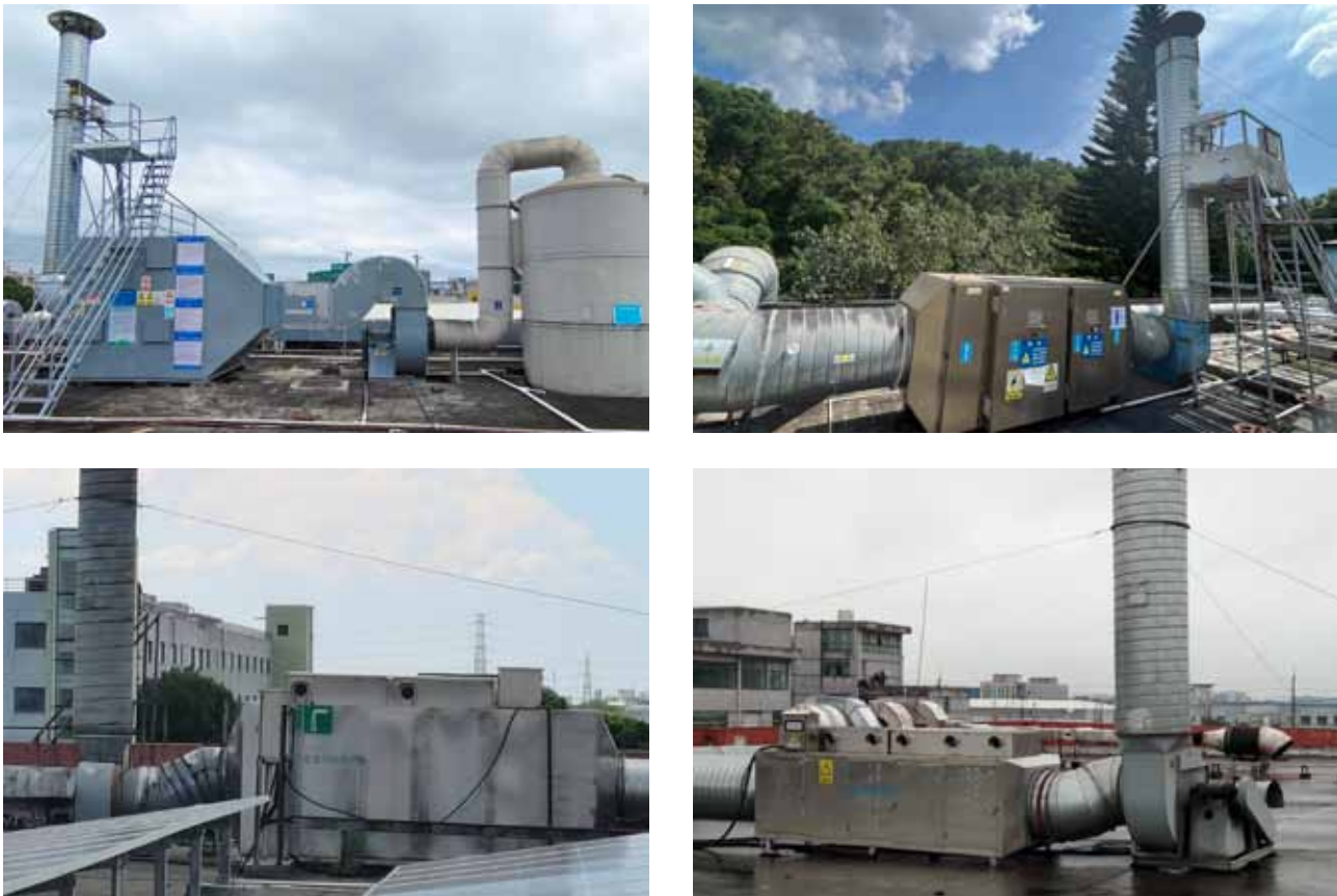
Waste gas treatment equipment of various companies
