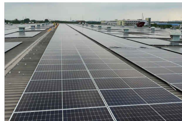
Photovoltaic project at C & C's Shanghai base
