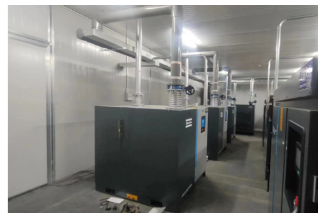
Central low-pressure air supply
