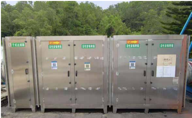
Secondary activated carbon treatment equipment
