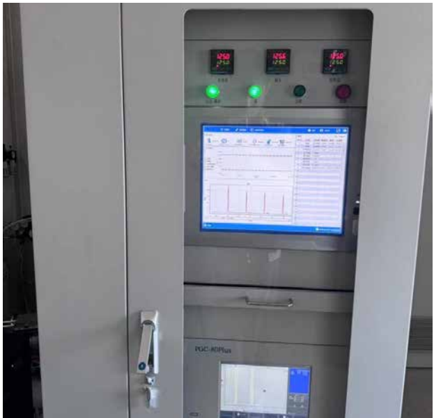
VOCs monitoring equipment (C & C Guangdong)
