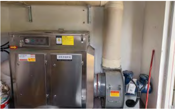
Activated carbon adsorption equipment
